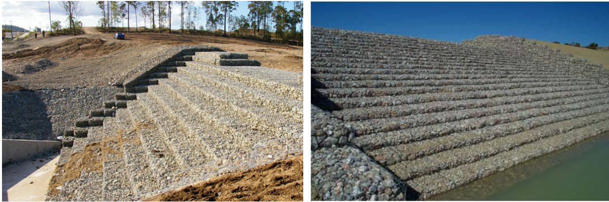
Fig. 25. Gabion protections at Pacific Pines (left) and West Cornfield (right) Dams (FEMA, 2014)
