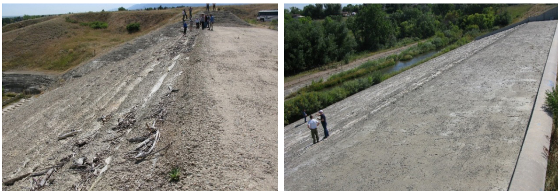
Fig. 47. Examples of RCC overtopping protection in the USA. Left: Left Hand Valley Dam. Right: Leyden Dam
