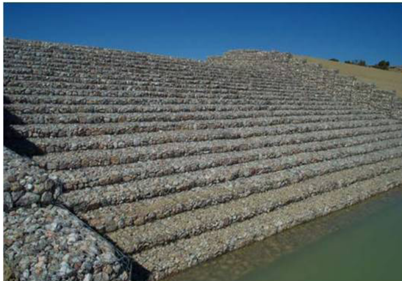
Fig. 4. Gabion lining of the downstream slope of the West Cornfield Dam (USA). (Photo: Tom Hepler)
