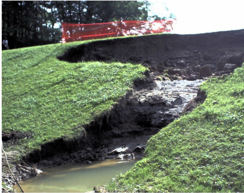
Fig. 7. Virginia Kendall Dam, Ohio, following three hours of overtopping with approximately 30 cm of hydraulic head above the crest. The slope of the dam was 2.5 (FEMA, 2014).
