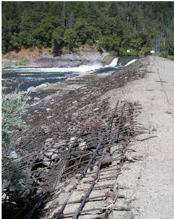
Fig. 21. View of the downstream slope of the Pit No. 7 Afterbay dam (FEMA, 2014)
