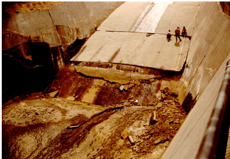
Fig. 55. Breaking of the slabs of the spillway channel of the Big Sandy Dam (Photo: William Fiedler)
