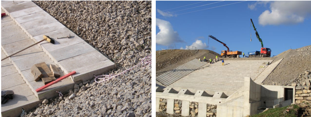
Fig. 42. Barriga Dam. Left: Laying the cable through the holes of the WSBs. Right: Transporting the WSBs to the site by mobile cranes using steel bars inserted into the cross hole.
