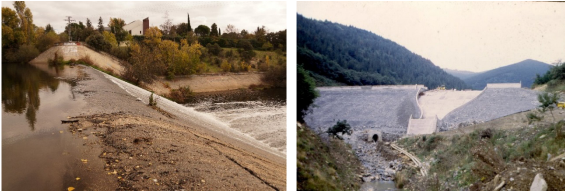
Fig. 52. Spillways with concrete slabs in the dam body. Left: Molino de la Hoz Dam. Right: Llodio Dam (Spain)
