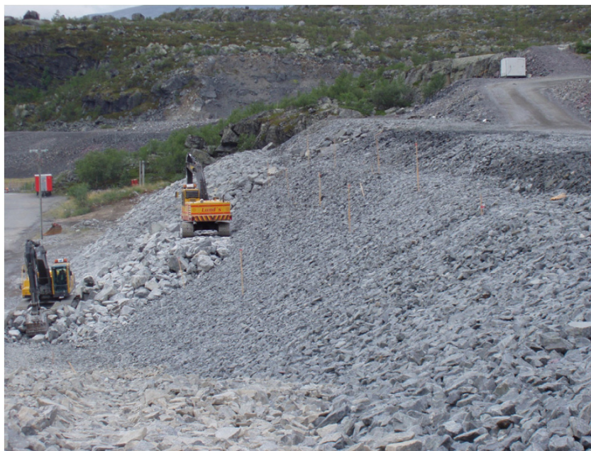
Fig. 19. Construction of the rockfill toe berm at Suorva Dam in Sweden (Nilsson & Rönnqvist, 2004)
