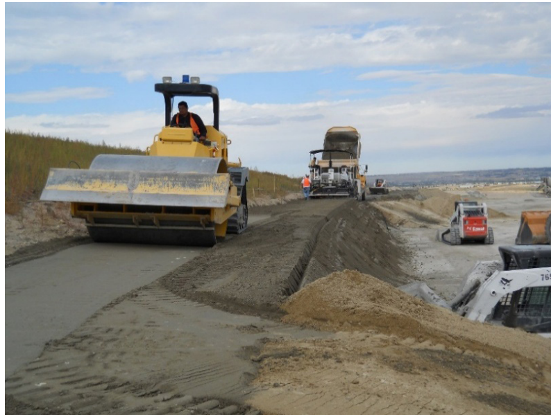
Fig. 34. Installation of cement soil protection (Photo: Korey J. Kadrmaz and Robert J. Huzjak)
