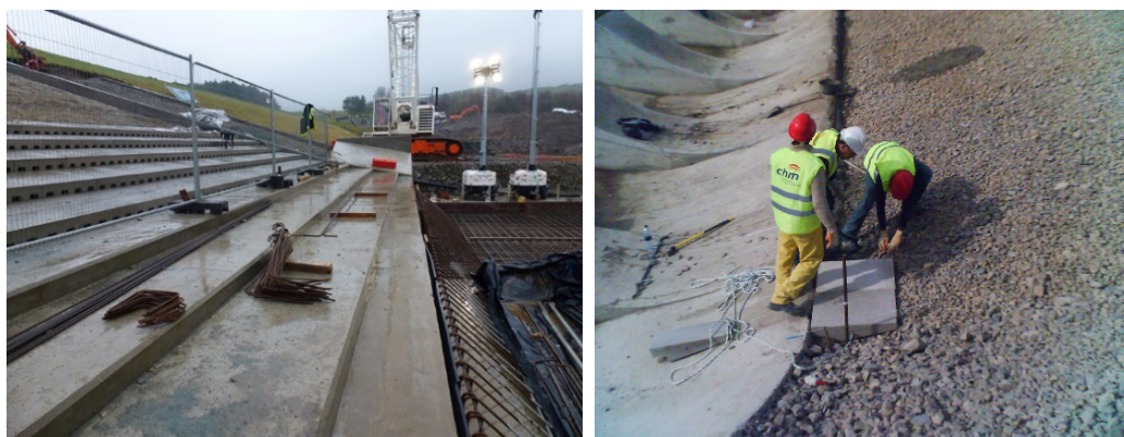
Fig. 44. Left: Support structure at the downstream end of the chute of the Odgen Dam (photo: P. Thurlwell. Pascoe, P&S Consulting Engineers, Ltd.). Right: Placement of the first row of blocks supported on the flip bucket of the Barriga Dam
