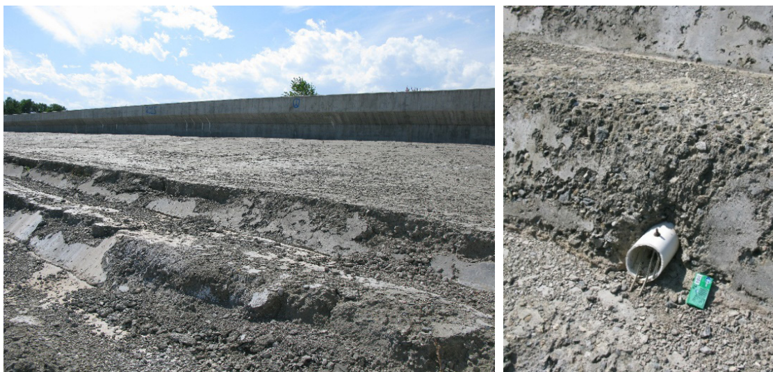
Fig. 48. Leyden Dam. Left: Inlet structure with spillway wall and stepped chute, seen from downstream. Right: Exit of one of the drainage conduits in the stepped slab of the chute.
