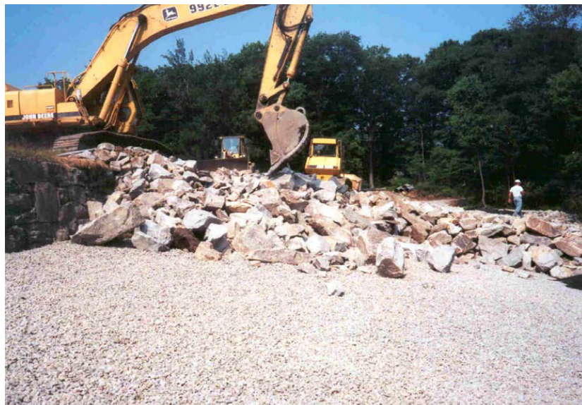
Fig. 12. Installation of a riprap protection in Upper Stoneville Dam, USA. (Photo: Thomas Hepler)
