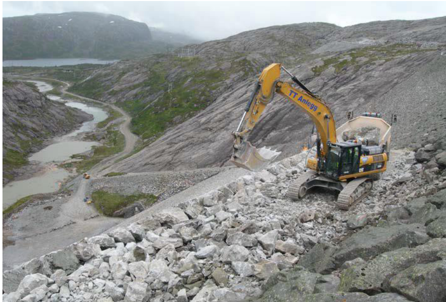
Fig. 13. Installation of a breakwater protection placed in Svartevatn Dam, Norway. (Photo: Priska H. Hiller)
